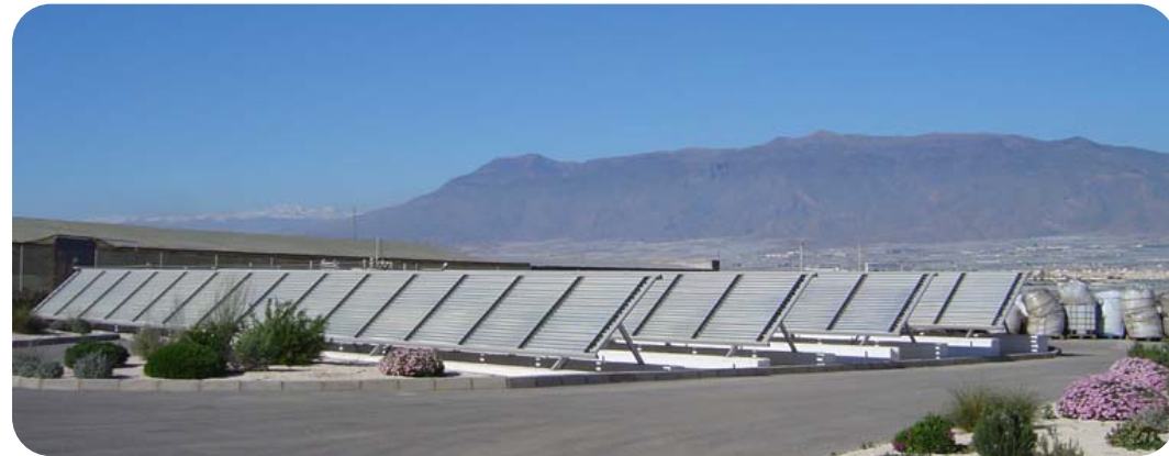
150 m 2 CPC detoxification plant, Almería, Spain
