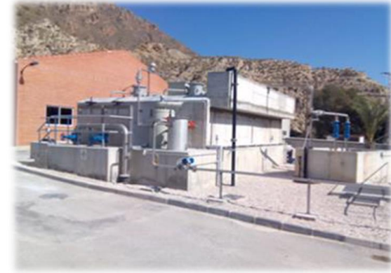
Anaerobic bioreactor (700 m 3 /day)
