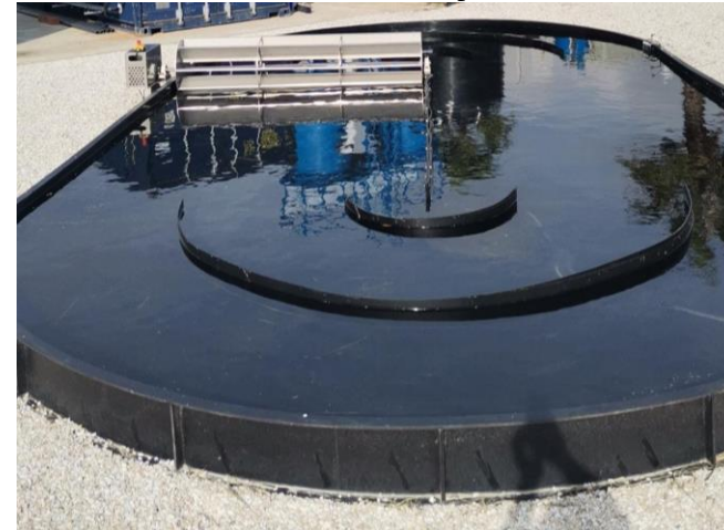
Automatic demo plant 37 m 2 (7.4 m 3 )
