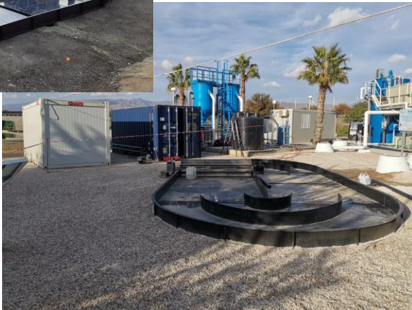
Raceway Pond Reactor Vessel
