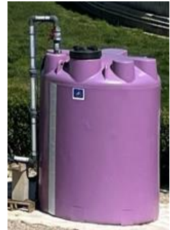
E Storage tank
